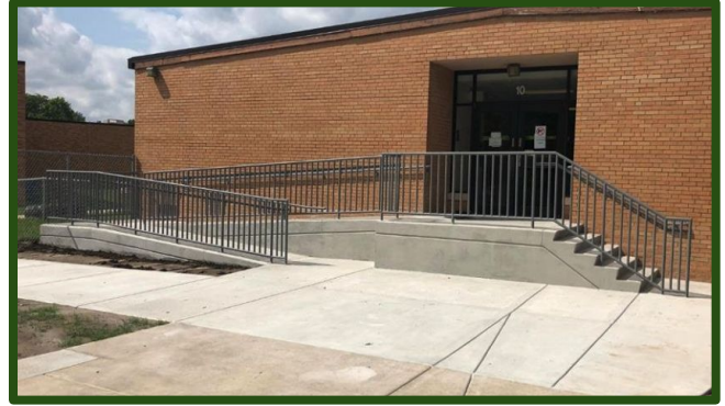
Swaney Elementary students and staff have a new accessible ramp to get to their playground!
